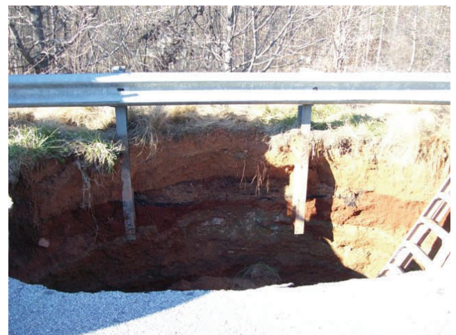
The 20 ft. X 30 ft. Sinkhole on I-85 Southbound at MM 178 in Georgia, at the South Carolina/Georgia state border.
